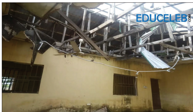
Figure 3: A dilapidated office within the administrative block of the Almajiri Model School, Dutsin-Ma. Source: Amoo (2019). Educeleb.com
